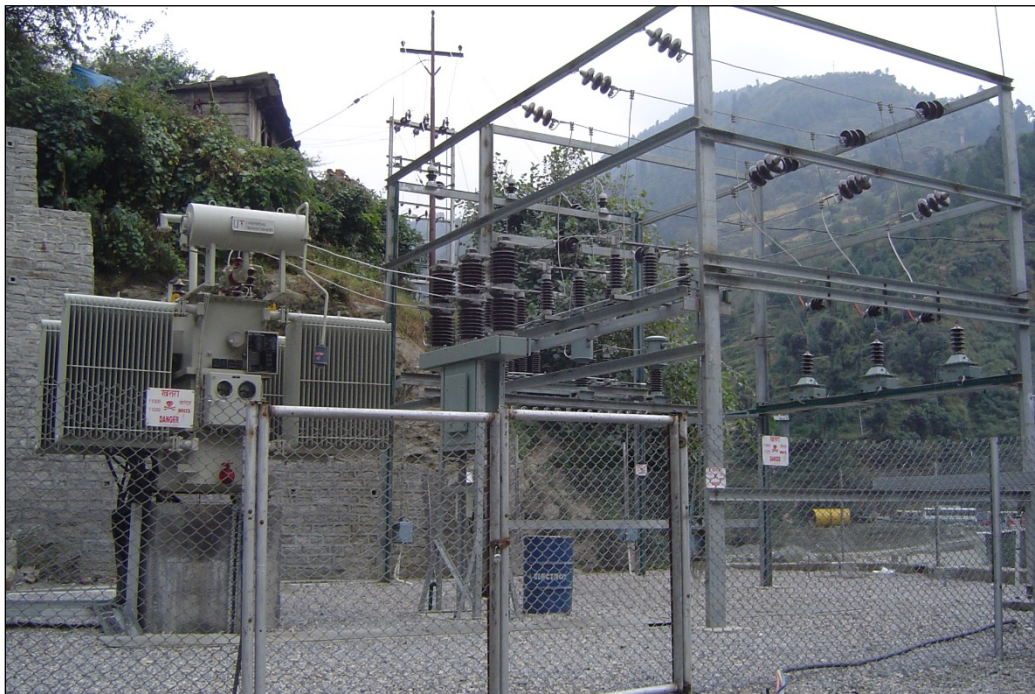
Photo of the switchyard
