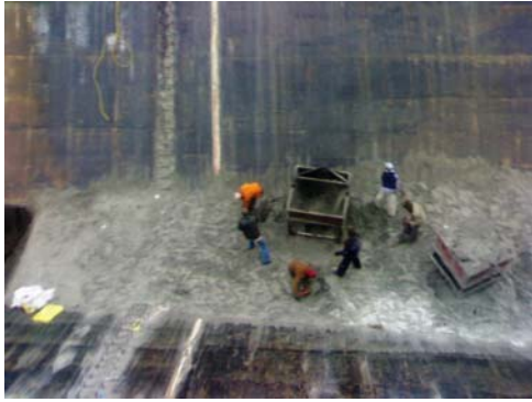
Silt deposition at Baspa site
