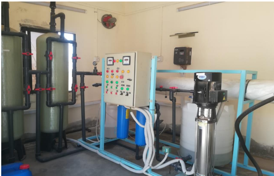
Figure 5: RO filtration plant for safe drinking water
