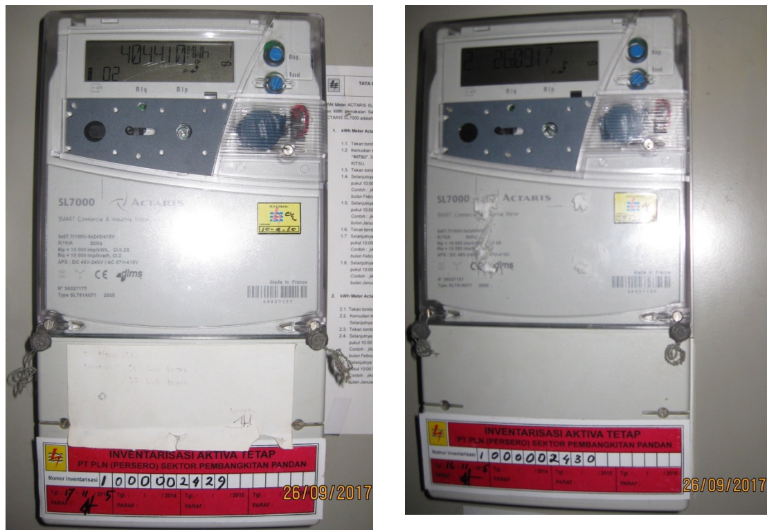
Figure 2 - Picture of main meters
