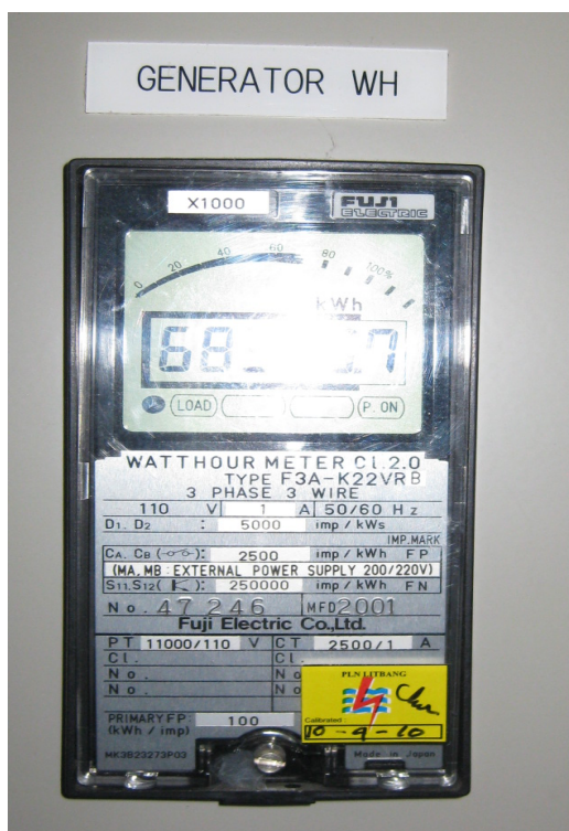
Figure 3 - Picture of main meter and production meter
