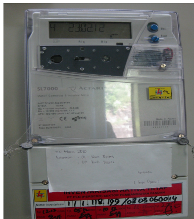
Figure 3 - Picture of main meter
