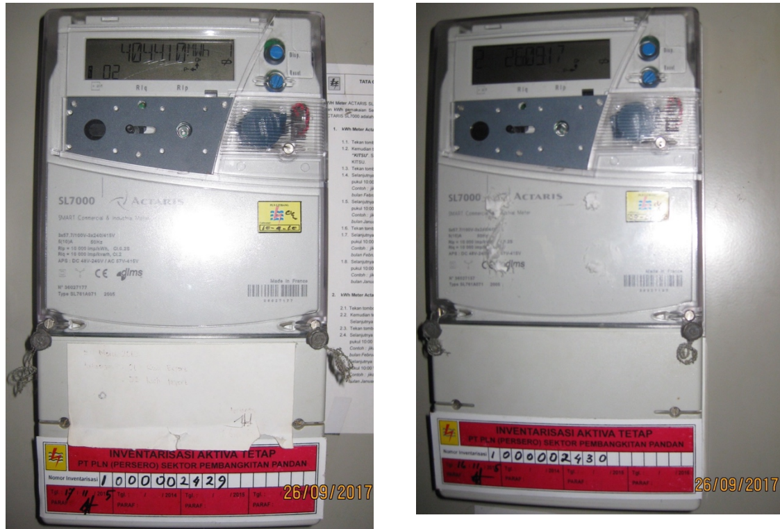
Figure 2 - Picture of main meters
