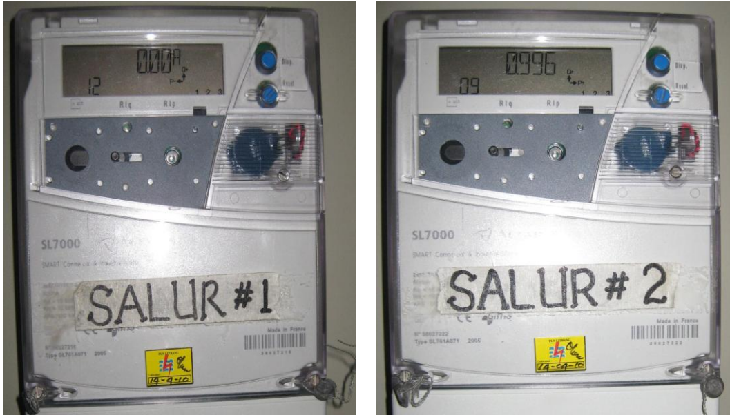
Figure 3 - Picture of main meter
