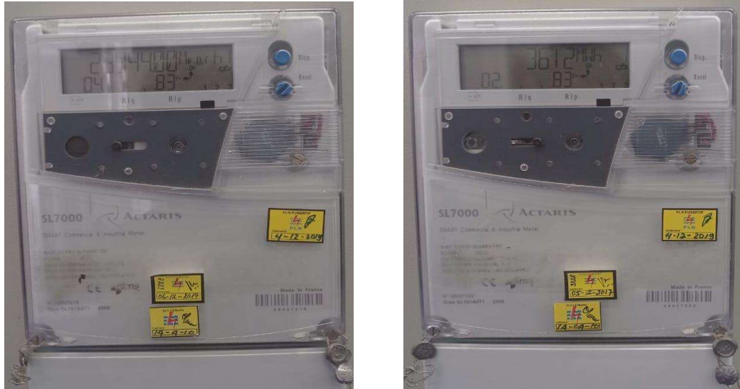
Figure 3: Pictures of main meters of Unit 1 (left) and Unit 2 (right)
