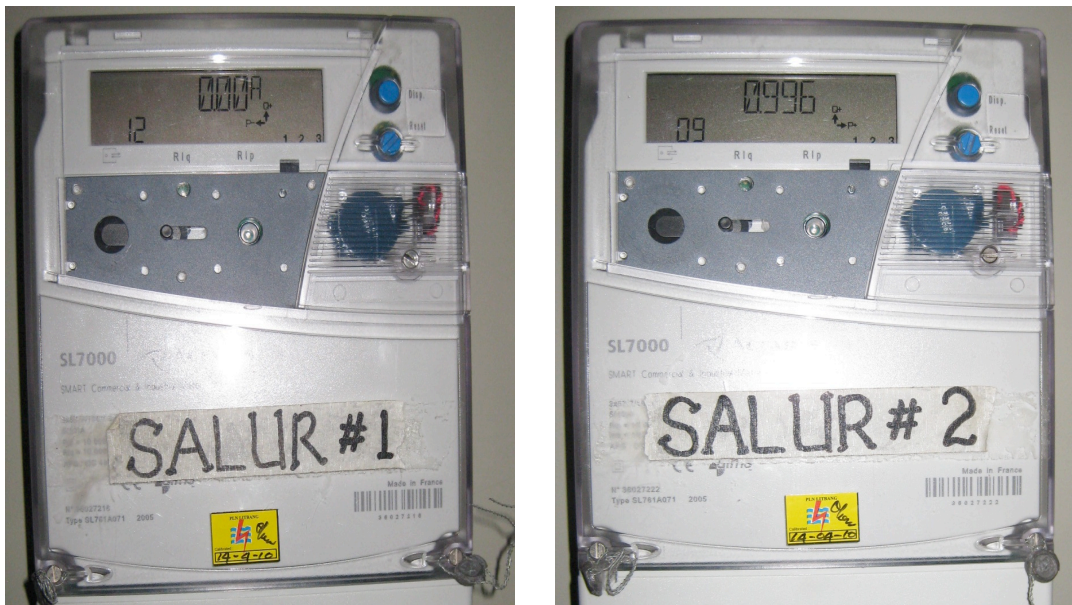
Figure 2 - Picture of main meter
