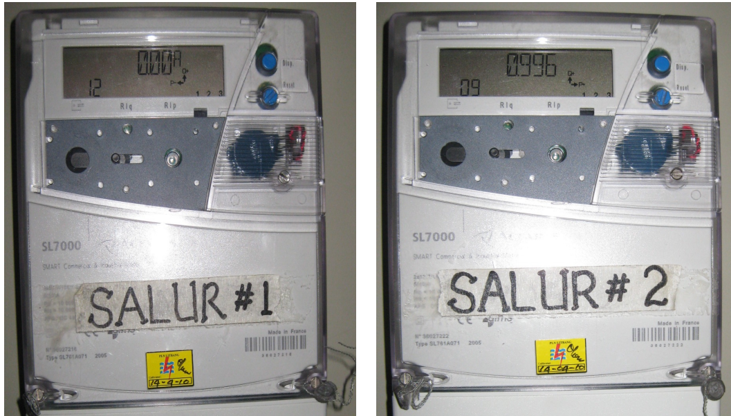
Figure 3 - Picture of main meter
