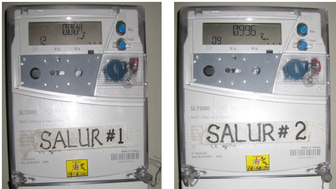
Figure 2 - Picture of main meter
