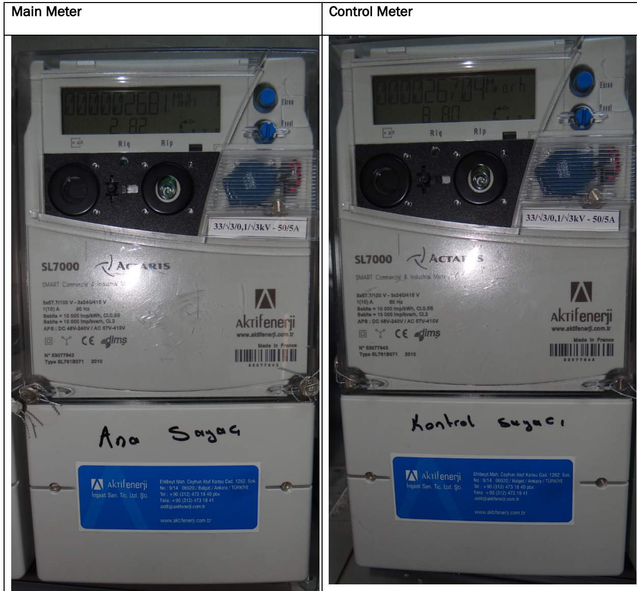
Figure 3: The pictures of the meters that measures internal consumption when the power plant is not operational.
