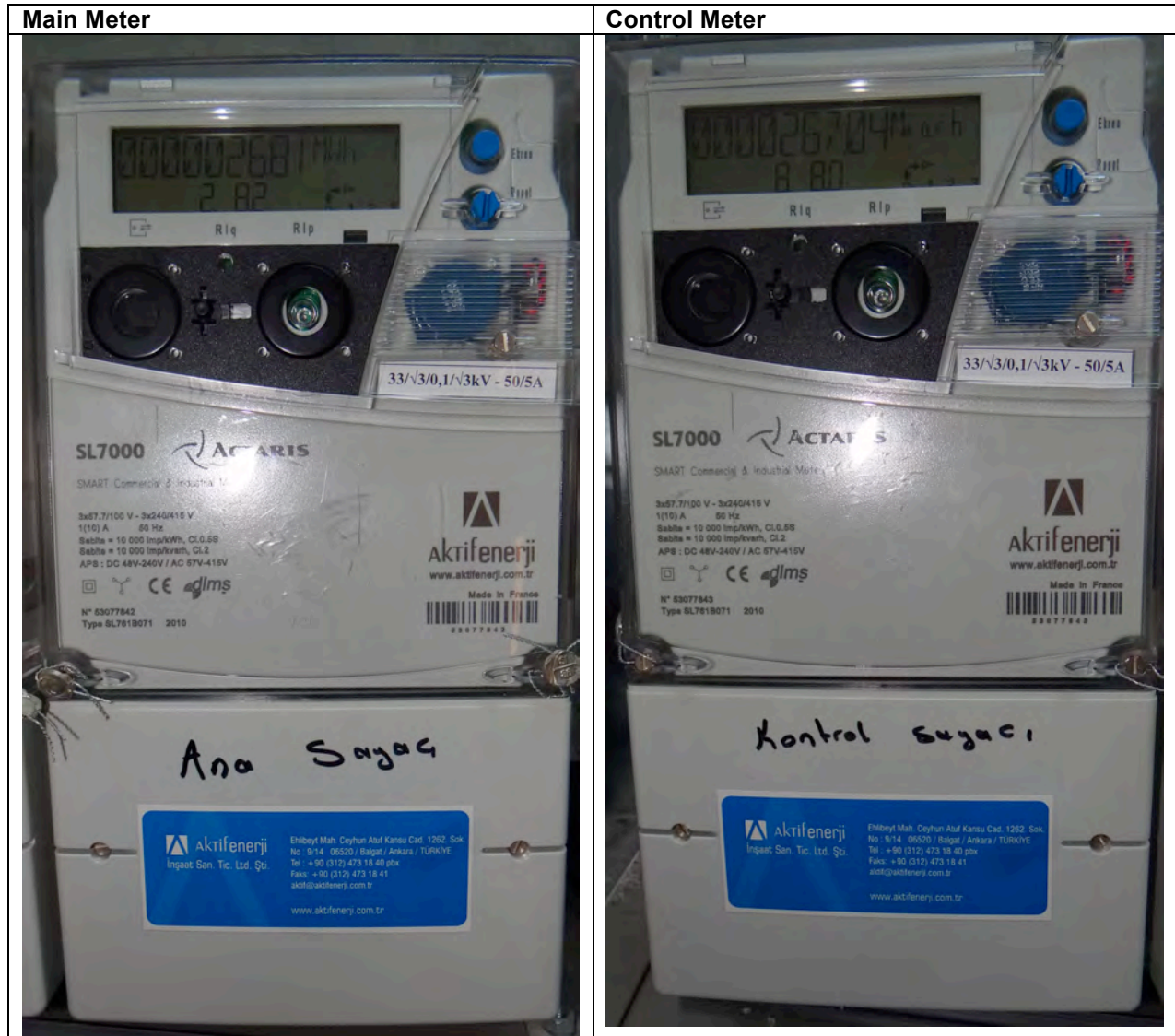
Figure 4: The pictures of the meters that measures internal consumption when the power plant is not operational.
