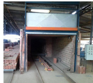
Figure 5: New Tunnel kiln which is being finalized at São Sebastião Ceramic.
