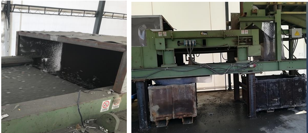
Picture 13 & 14: Components of eddy current separation installation
