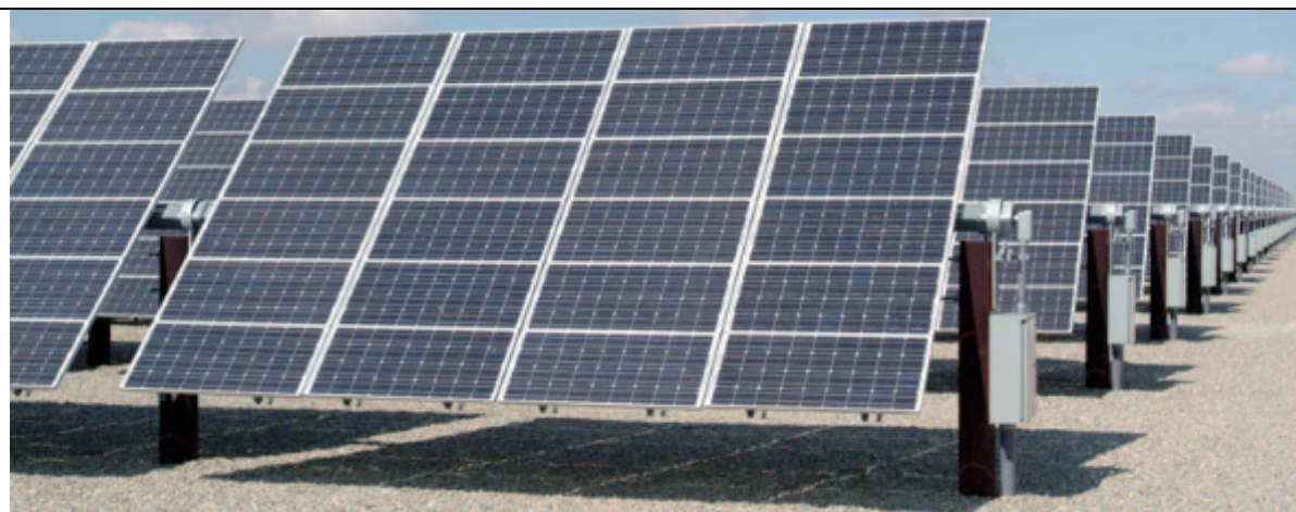
Figure 1: Mounting structure of the CPA
