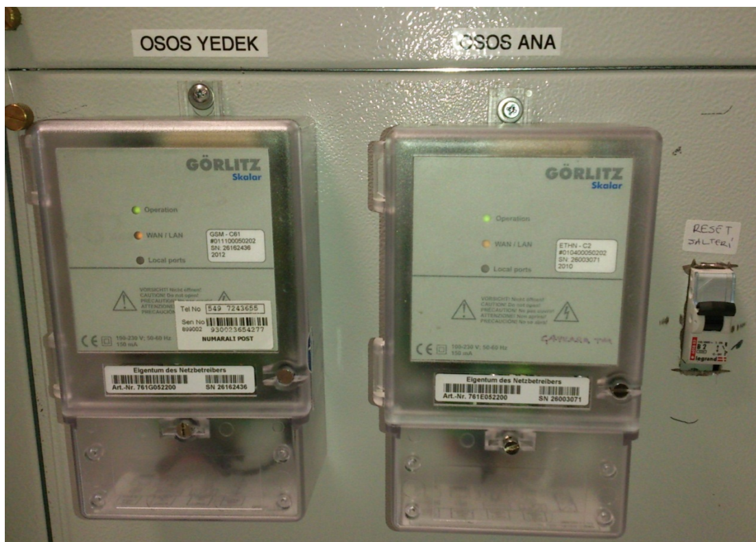
Figure 4: OSOS system installed in the meter control cabinet
