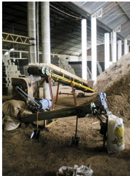
Figure 8. Biomass being processed to used as fuel in Eliane Ceramic.
