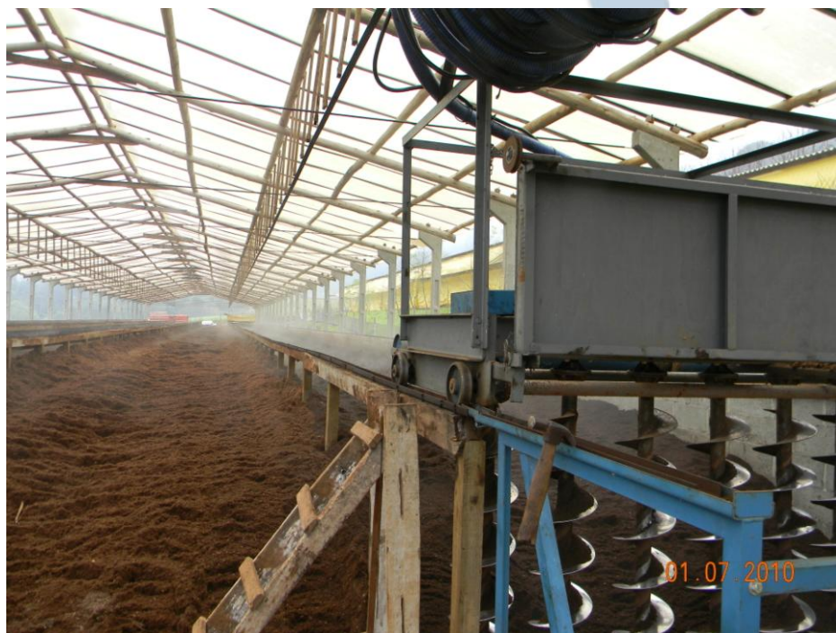
Picture 3. UMAC installation in Ramella's swine farm
