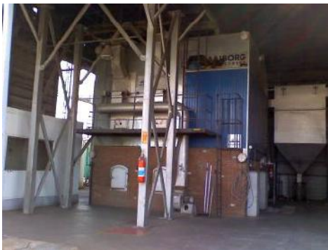
Boiler using renewable biomass at both sites of the project
