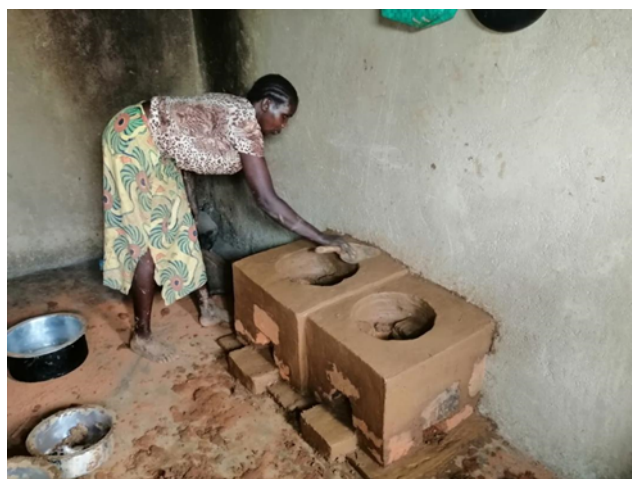
Figure 3 The energy efficient cook stove being installed in a household kitchen by a female Artisan.
