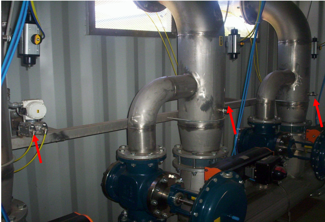
Figure 1. Backup flow meters
