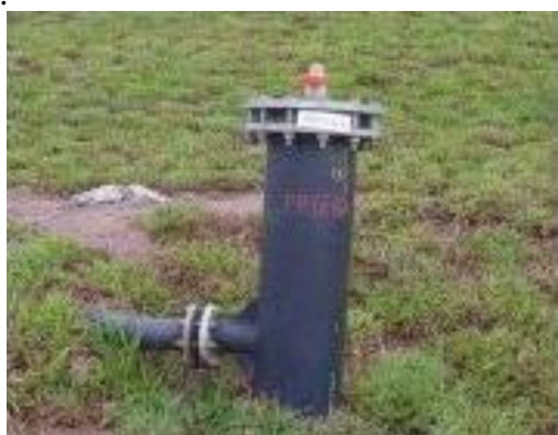
Figure 3 – Example of wellhead (source: Biogás Ambiental 2 )
