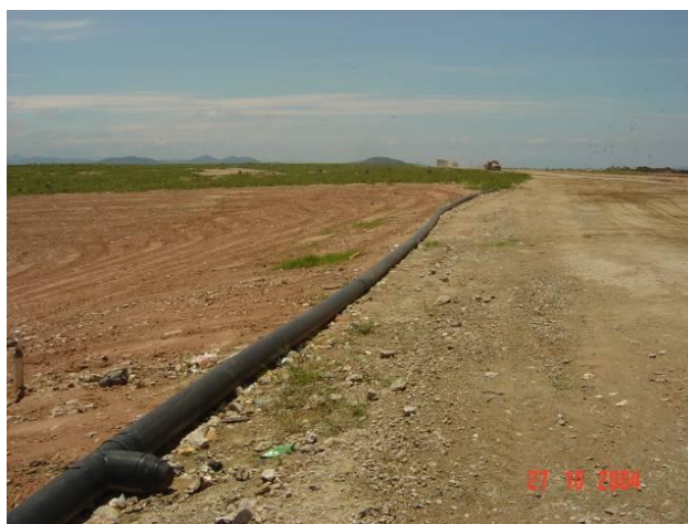
Figure 6 – Example of a transmission pipeline
