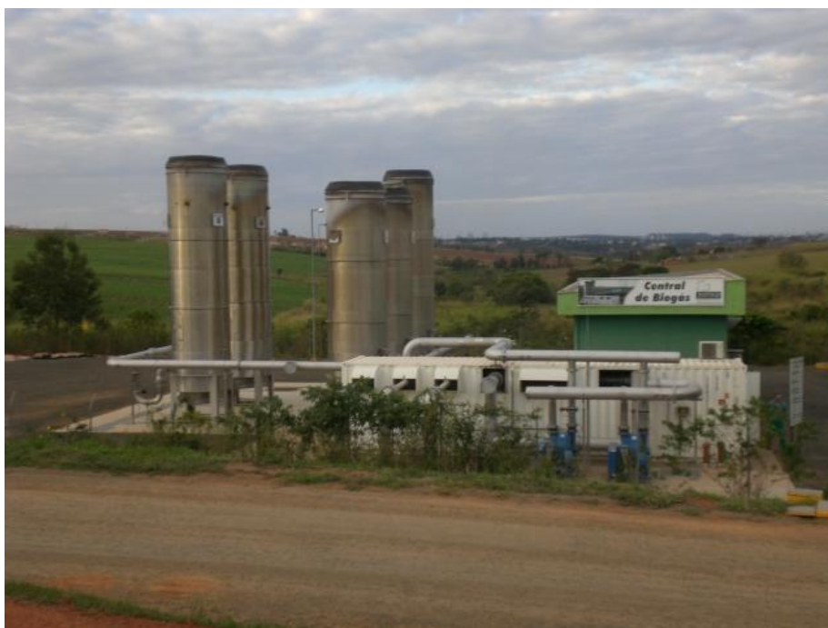
Figure 7 – Biogas facility (source: ESTRE Ambiental)
