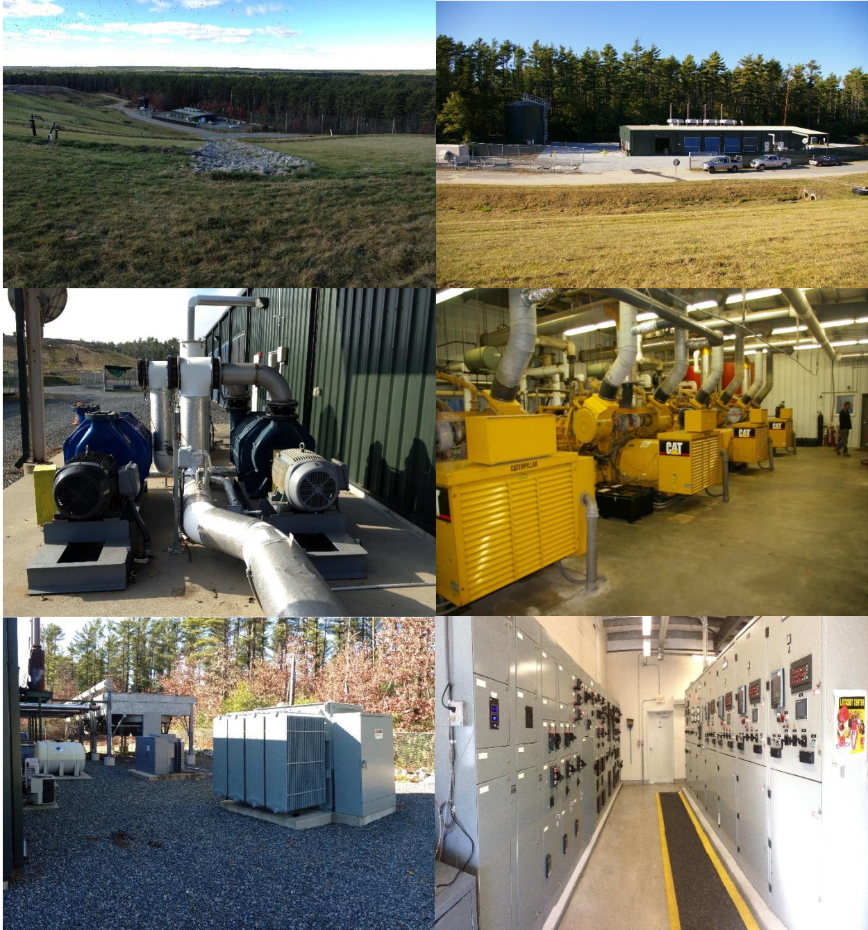
Figure 1: The Project – row 1: LFG piping and Project facilities; row 2: LFG pumps and electric power generating equipment; row 3: transformer and control room
