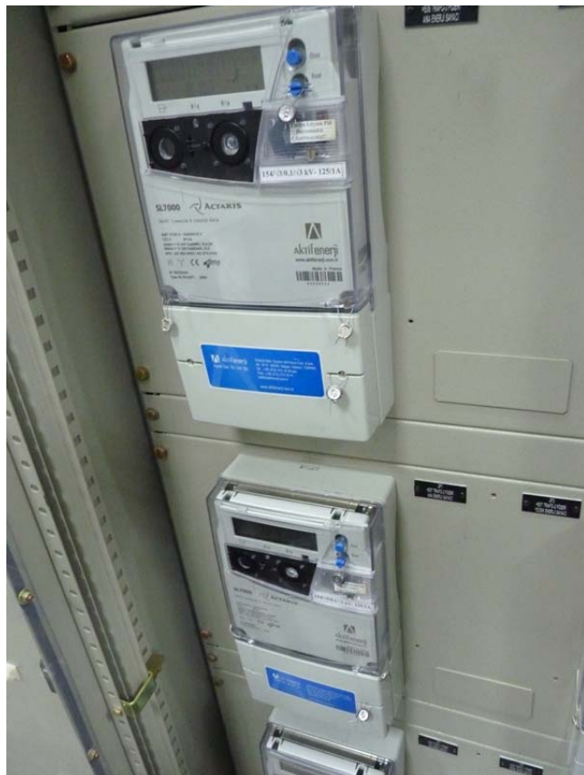
Figure 2: Primary meter2 at the plant (sealed for optical port)
