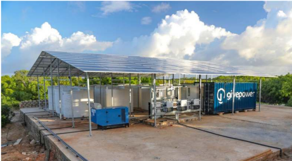
Figure 5: Solar powered desalination plant
