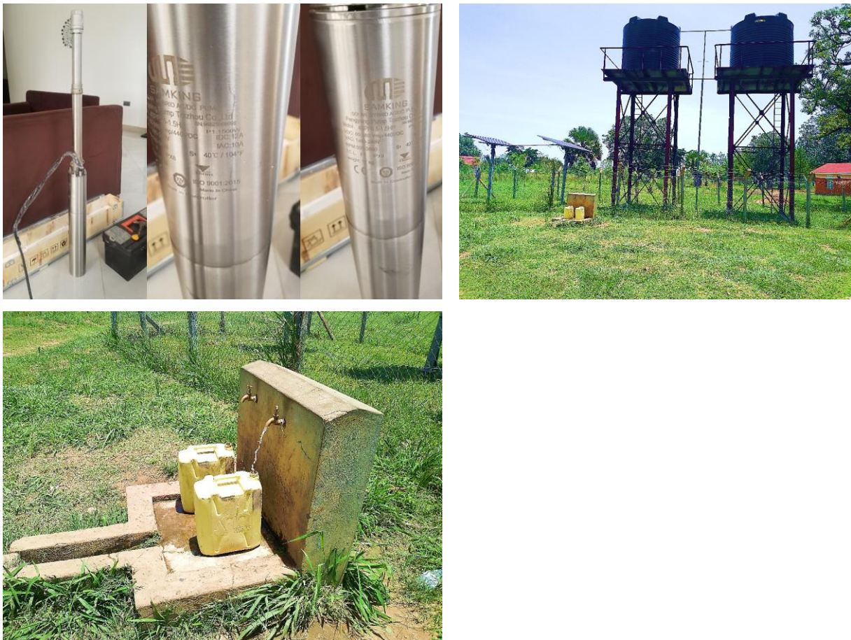
Figure 5: Photos showing the pump model, solar panels and water storage tanks, and distribution taps of the Omoro Solar Pump (LAN086).
