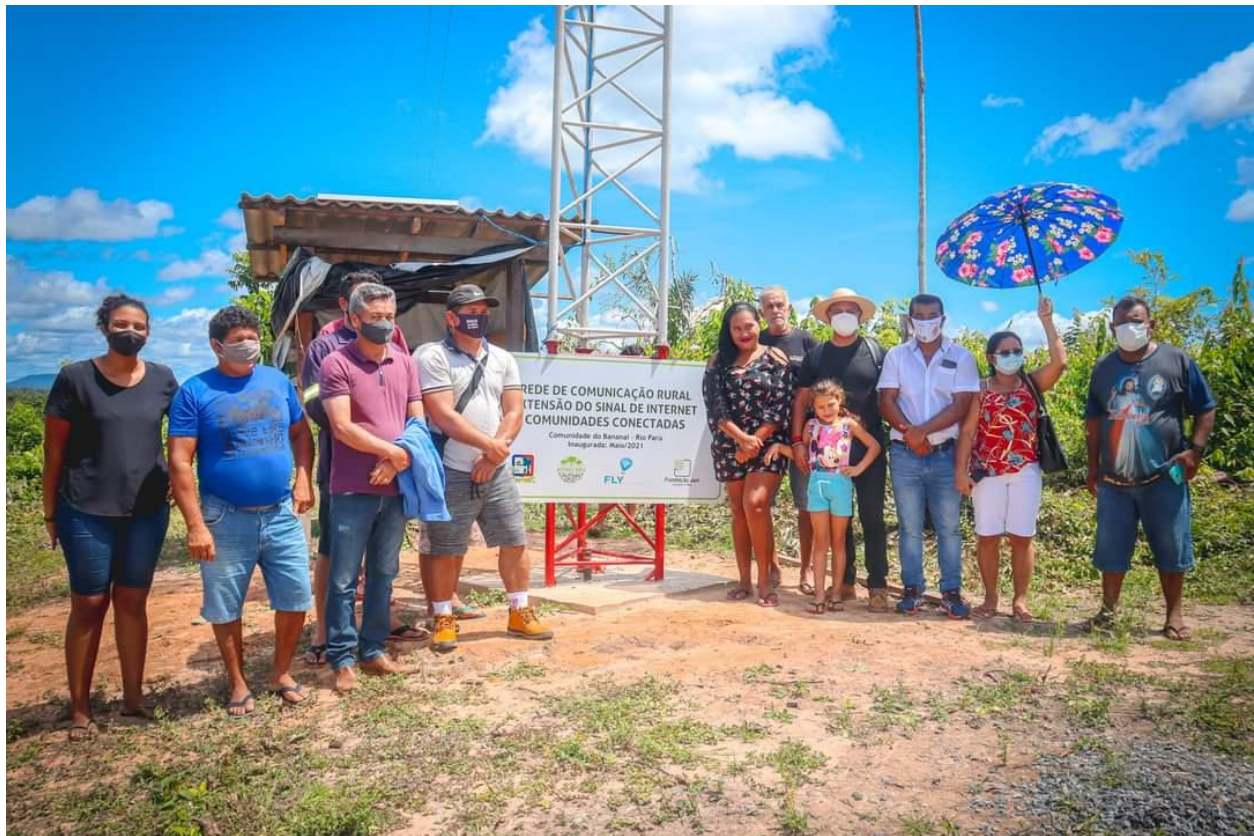
Figure 30. Rural communication tower (internet) installed in the Bananal community - Rio Parú.
