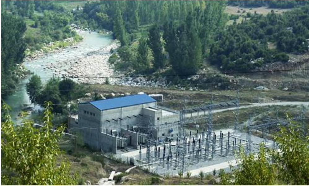
Figure 12. Power House and Switchgear Station
