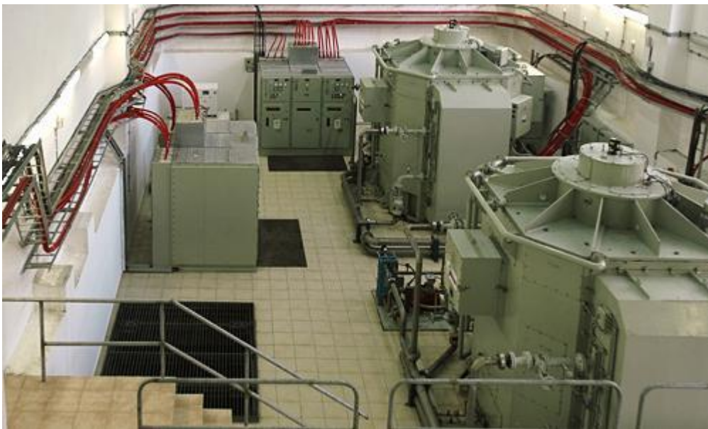
Figure 13. Power House Interior
