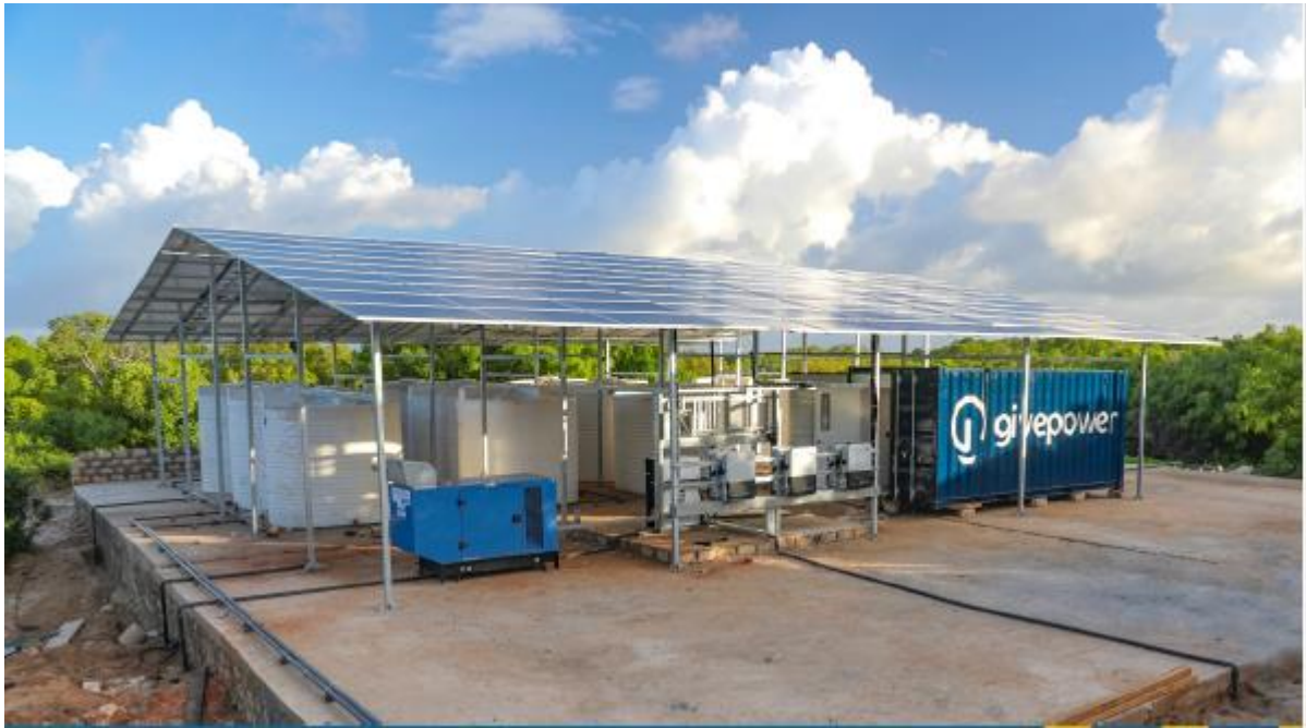
Figure 3. Photograph example of the GivePower MAXI plant.
