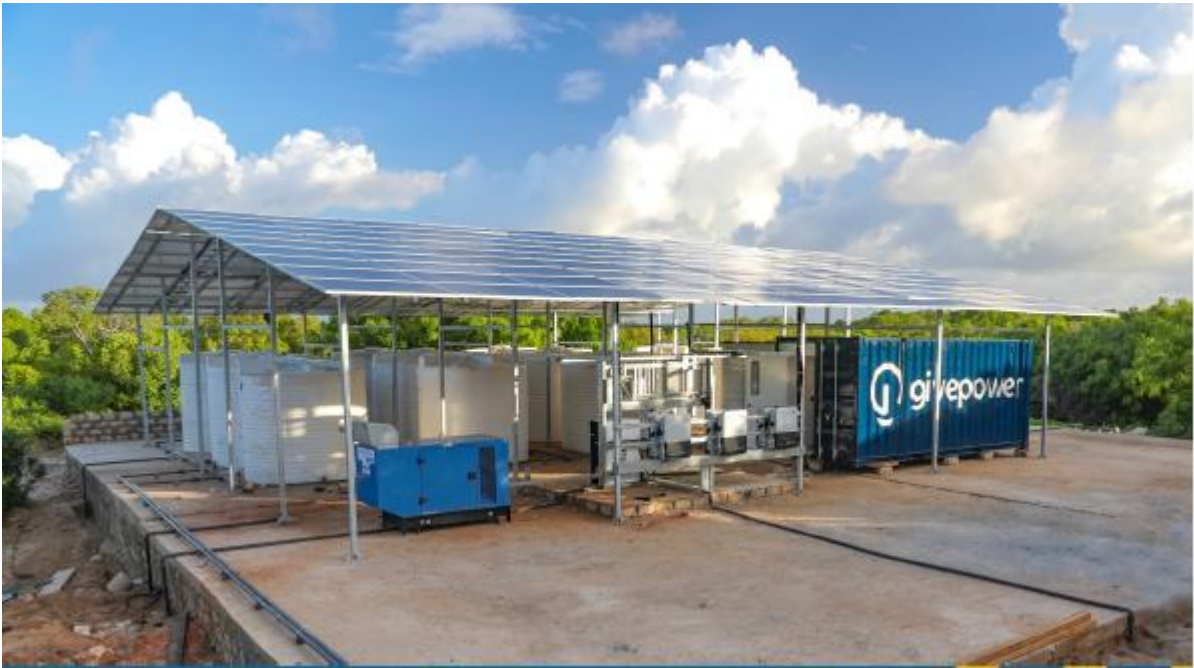
Figure 3. Photograph example of the GivePower MAXI plant.
