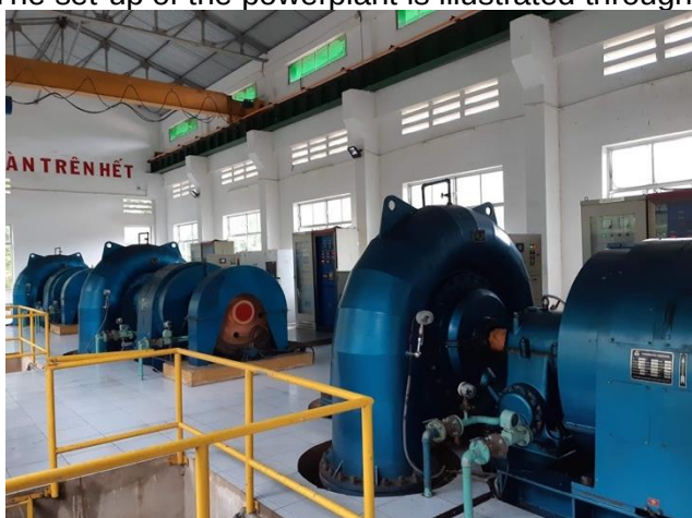
Pict. 1 Turbines & generators
