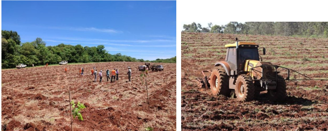
Figure 8. Site preparation in Garruchos Ranch for the plantation of native species (September 2022)
