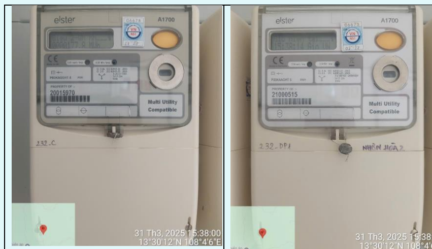
Main meter 232C Back-up meter 232DP1
