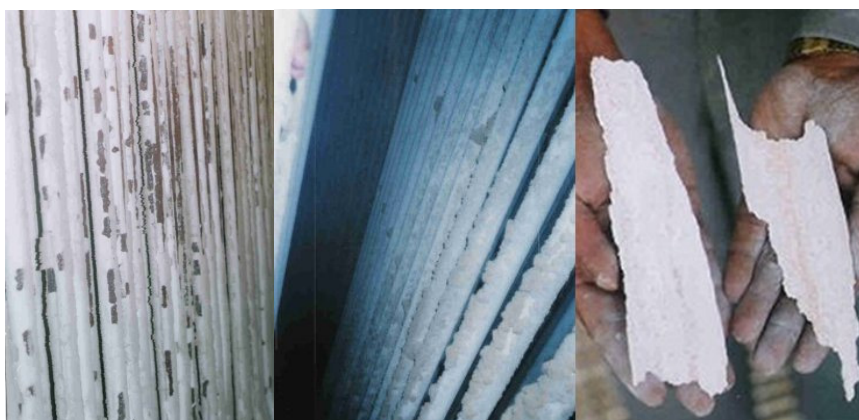
Figure B.2: Corrosion, deposits and scale formation on super-heater tubes
