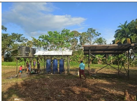
Water supply system. Berlin Community
