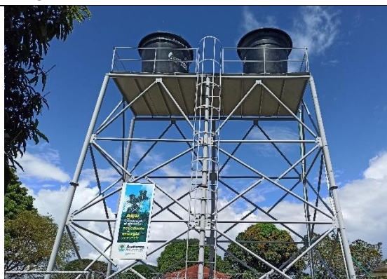
Water supply system. Sarrapia Community (120 families)
