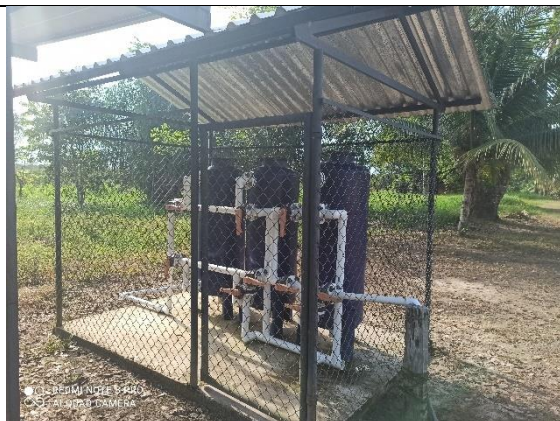
Water supply system. Manajua Community
