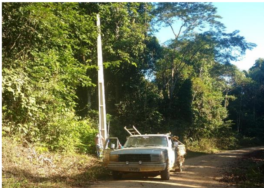
Figure 10 - Electrical network installation at RESEX Rio Preto-Jacundá
