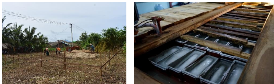
Figure 7: Construction of the ice plant (left) and Production of ice blocks (right)
