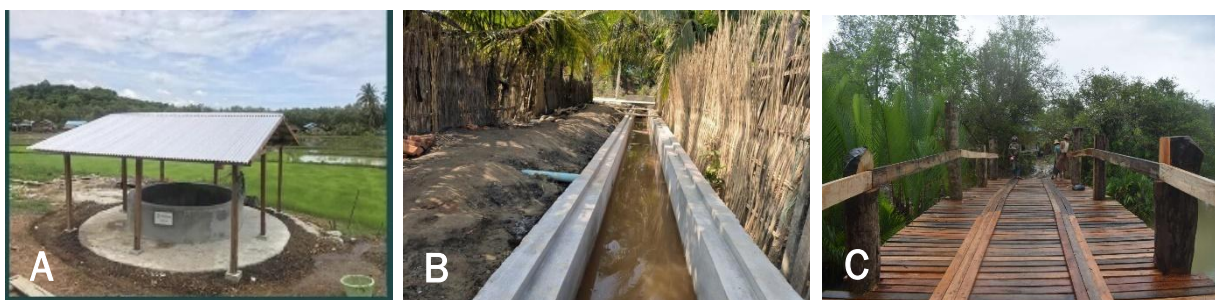
Figure 15: A. well digging and fencing construction at Ma Tha, B. box culvert and drainage construction at Ward 3 Shwe Thaug Yan, and C. bridge construction at Phone Soe village.
