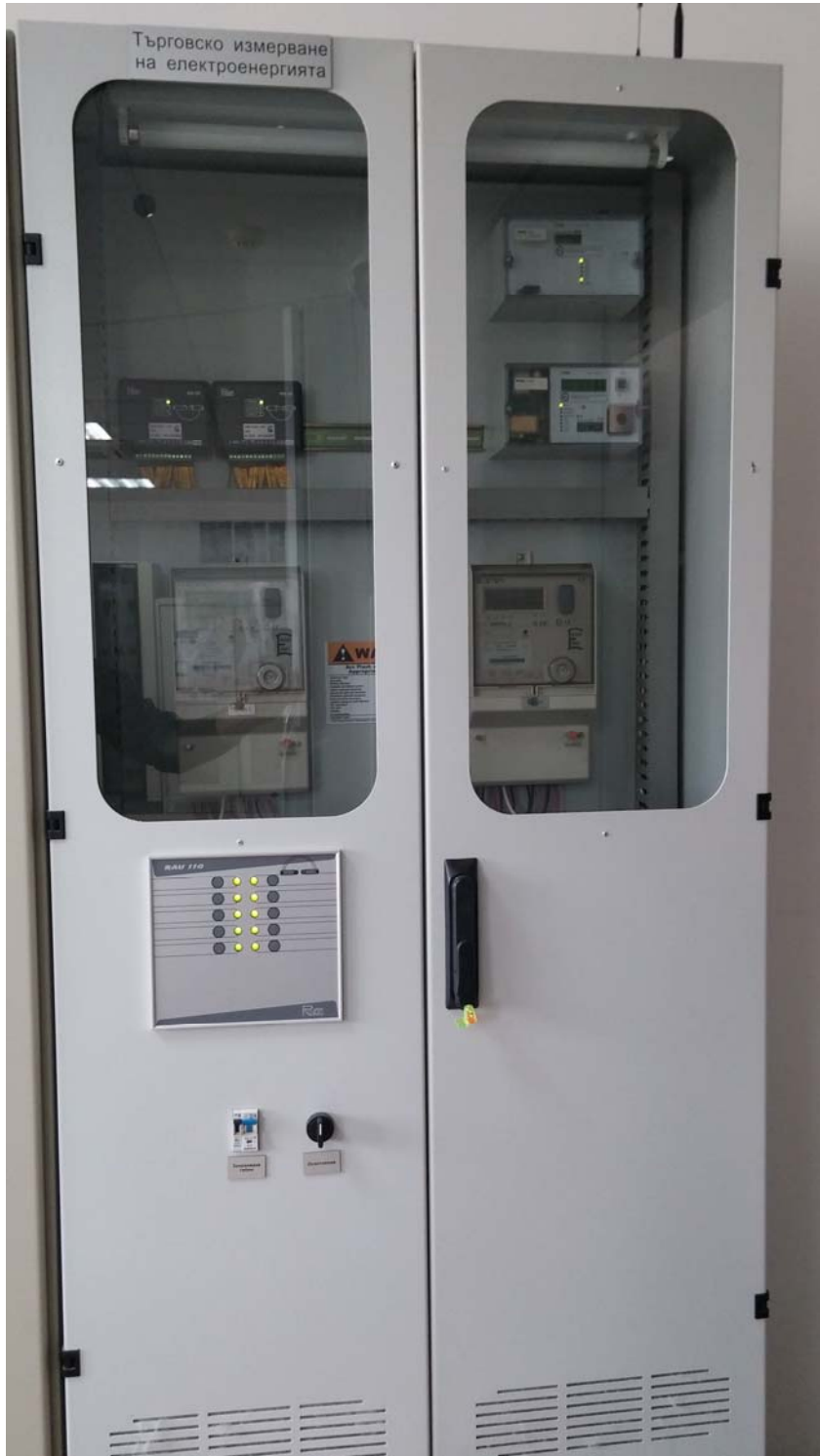
Fig 4: Commercial electric meters – control panel
