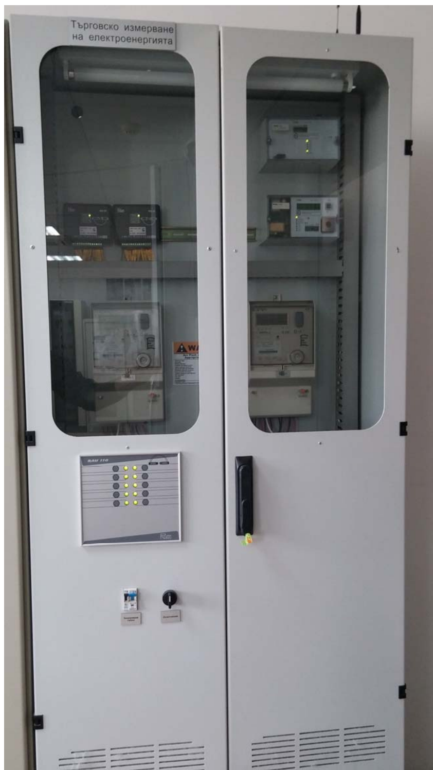
Fig 4: Commercial electric meters – control panel
