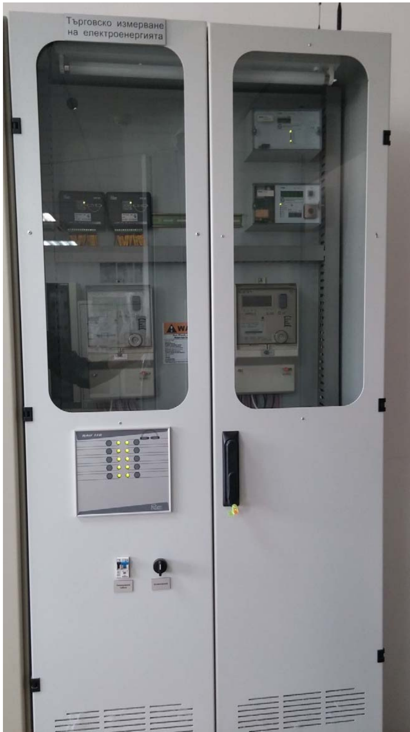
Fig 4: Commercial electric meters – control panel
