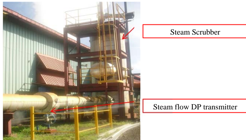
Figure 2: Location of steam flow transmitters (outlet of Unit's steam scrubbers).
