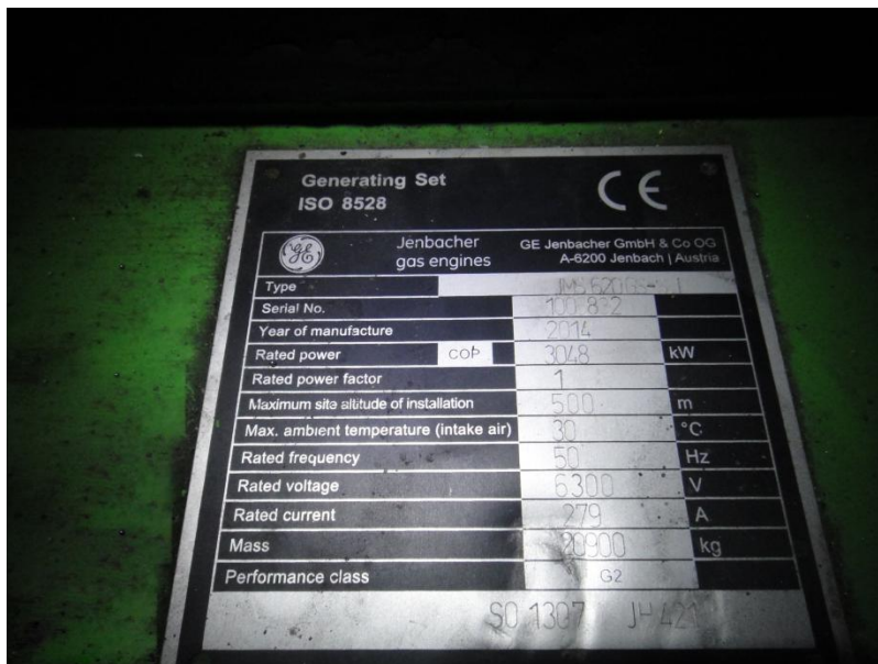
The nameplate of 2# Generators for Shanmushu CMM power plant
