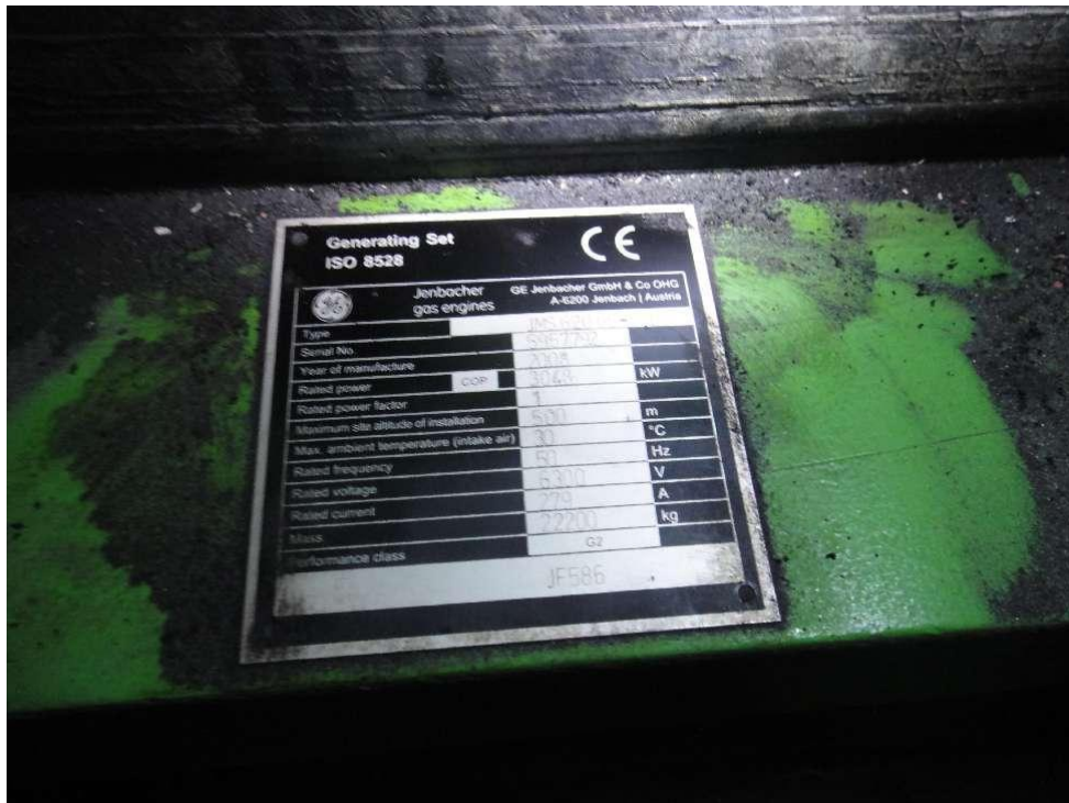
The nameplate of 2# Generators for Baijiao CMM power plant
