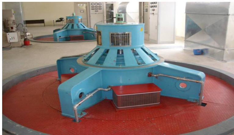
Figure 4: Photo of Kaplan Turbine
