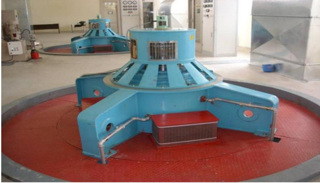
Figure 2: Photo of Kaplan Turbine
