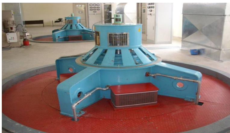
Figure 3: Photo of Kaplan Turbine
