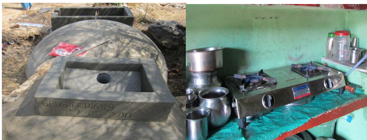
In construction Deenabandhu Biogas Unit in the project area and Biogas Stove in the kitchen
