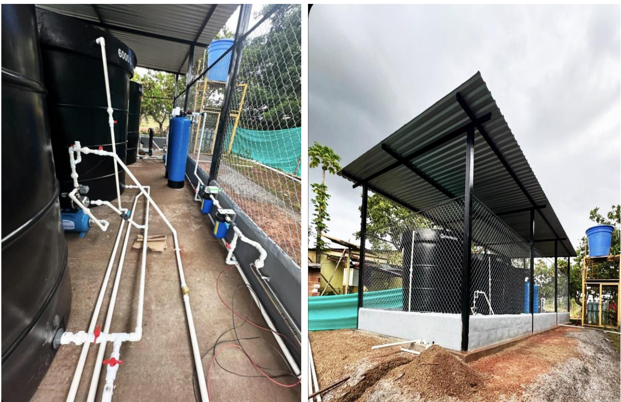
Figure 9. Drinking water plant for the primary school of La Esmeralda
